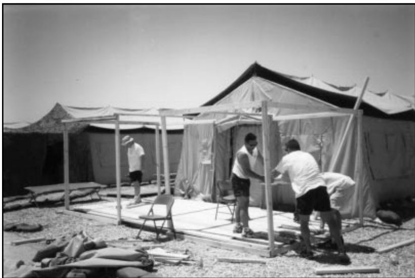
Members of the 4416th IS, Prince Sultan Air Base, Saudi Arabia, erect framing for camouflage netting to complete the deck they built in front of a squadron tent.
