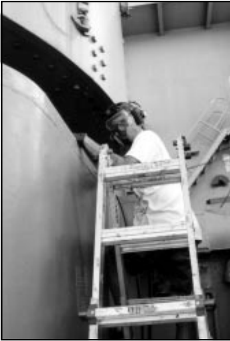
Master Sgt. David "Rusty" Strum lives up to his name as he chips away built-up corrosion.
